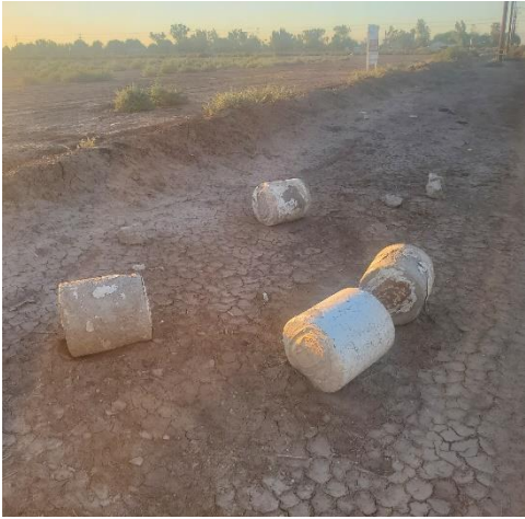
13. Concrete debris on west portion.
